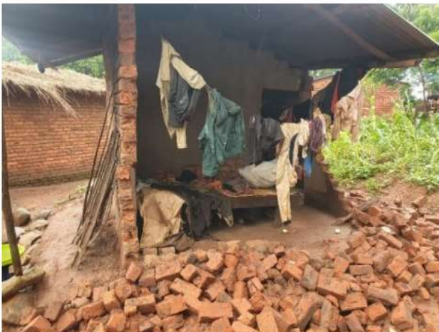
One of the many damaged houses in the area.
